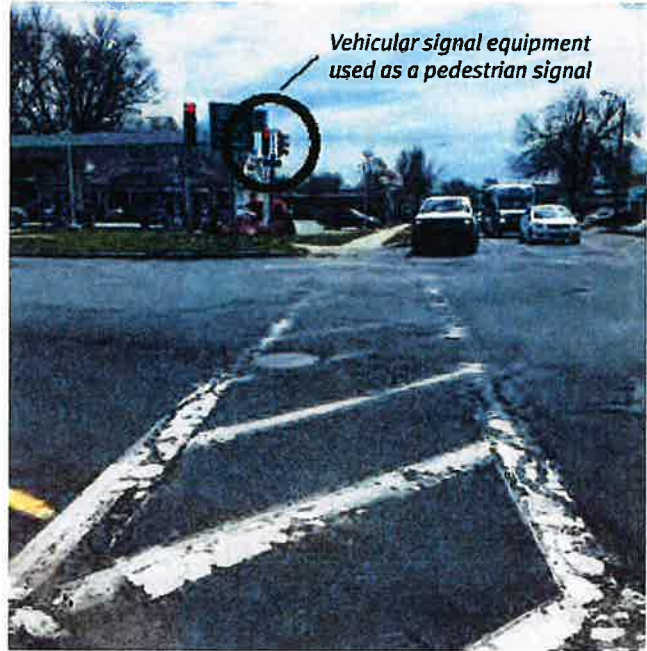
Park Avenue and Union Street intersection with long crossing distances and confusing pedestrian signal equipment
