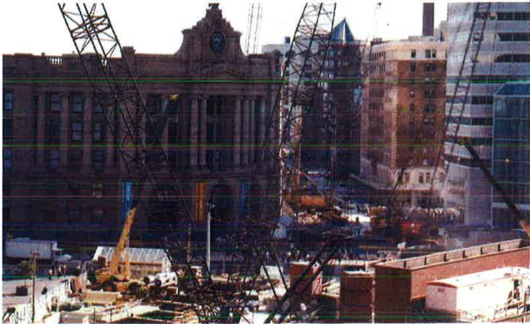
THE NORTHBOUND TUNNEL WAS AN IMPORTANT PART OF THE CENTRAL ARTERY/TUNNEL PROJECT, THE LARGEST URBAN INFRASTRUCTURE UNDERTAKEN IN U.S. HISTORY.
