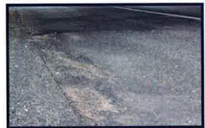
Figure 3 Drainage and Pavement Concern at Overpasses
