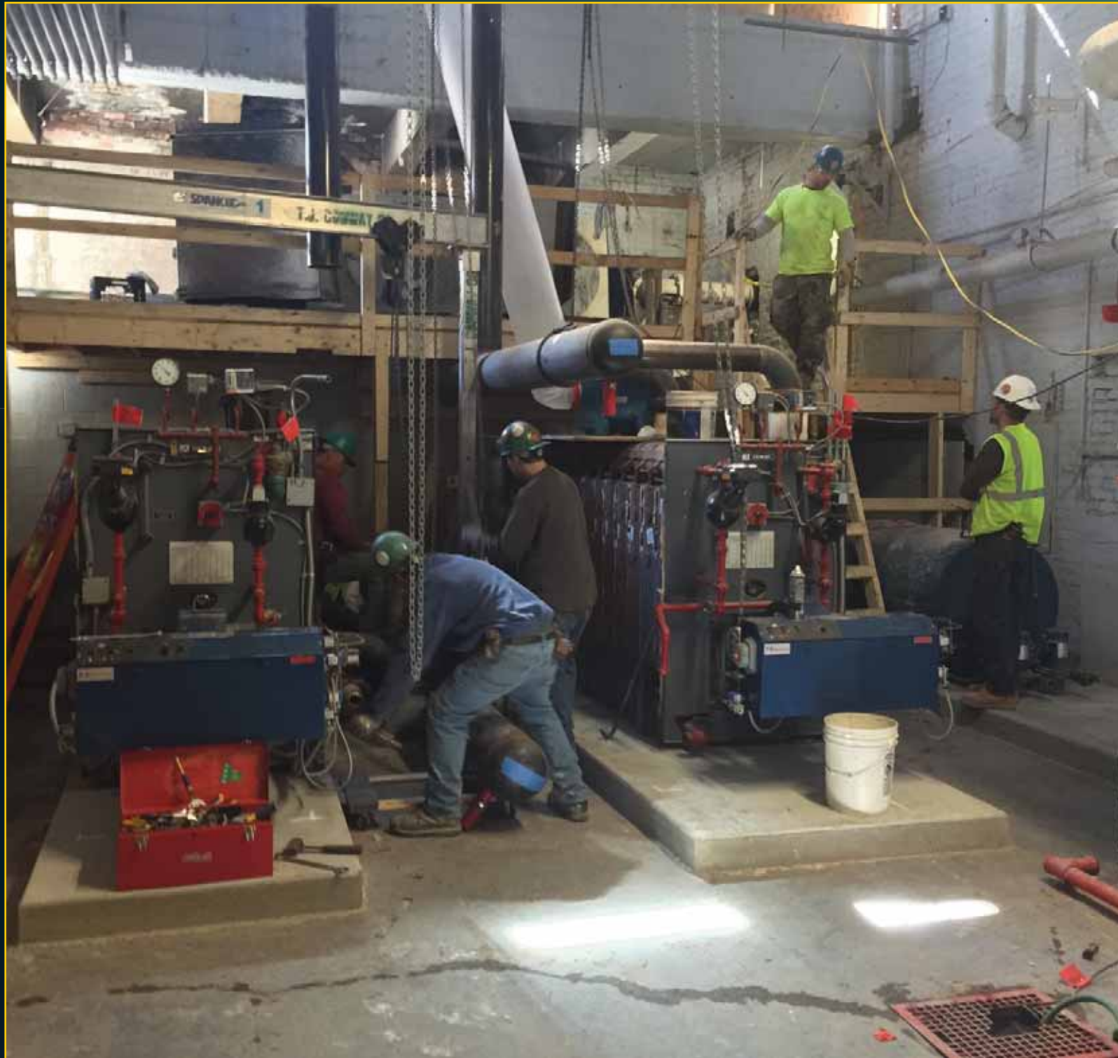
95 State Boiler Work - May 9, 2016
