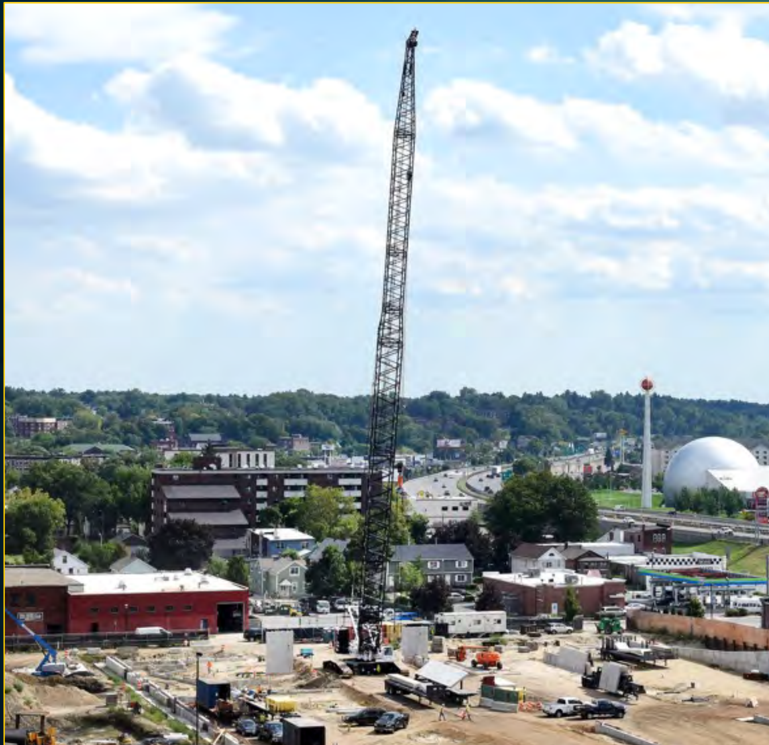
Garage Crane - September 14, 2016
