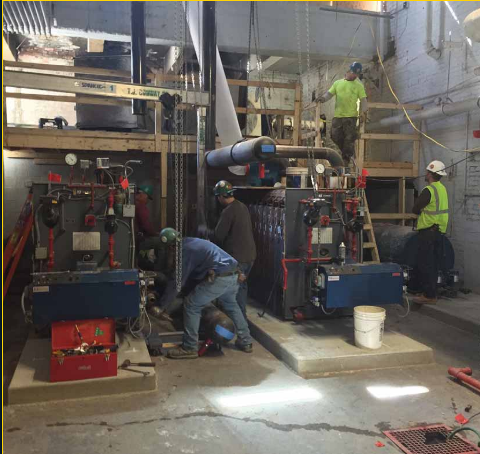
95 State Boiler Work - May 9, 2016
