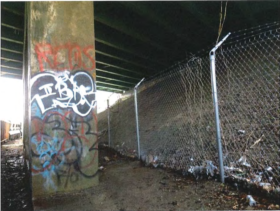
Figure 5 - Span beneath west side of the Rte. 16 overpass which could be re-graded to accommodate trail
