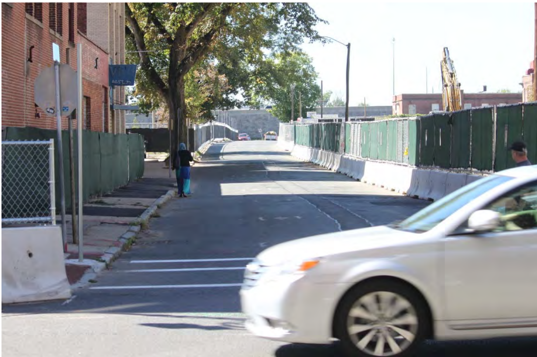
Figure 5. (Below) Pedestrian walking in street due to construction, blocked sidewalk and sidewalk irregularities.
