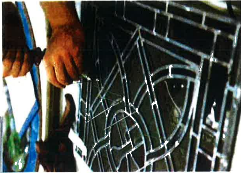
Flat support bars (above) or tie wires for round bars (right) are soldered to the window panel.
