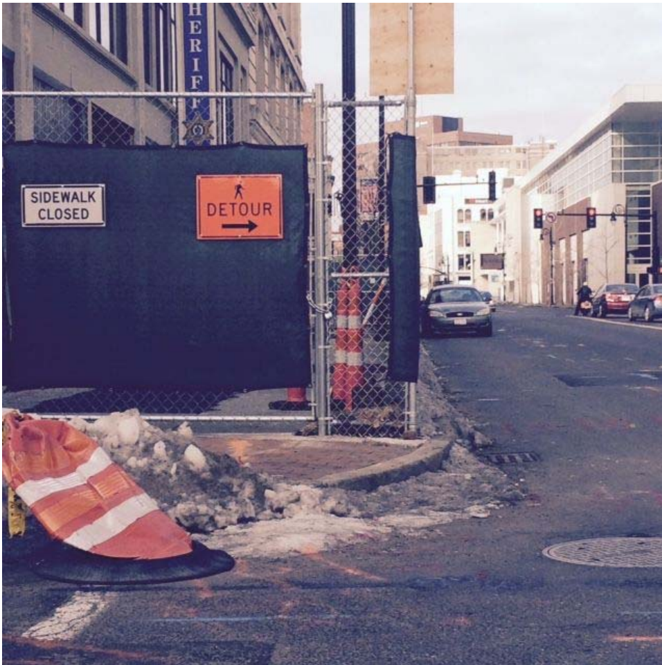
Figure 3. Main Street sidewalk is closed. The pedestrian detour sign directs people to walk in the street. This illustrates a street corner blocked by construction, snow and ice, with no handicap access.
