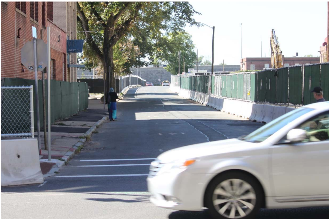
Figure 5. (Below) Pedestrian walking in street due to construction, blocked sidewalk and sidewalk irregularities.
